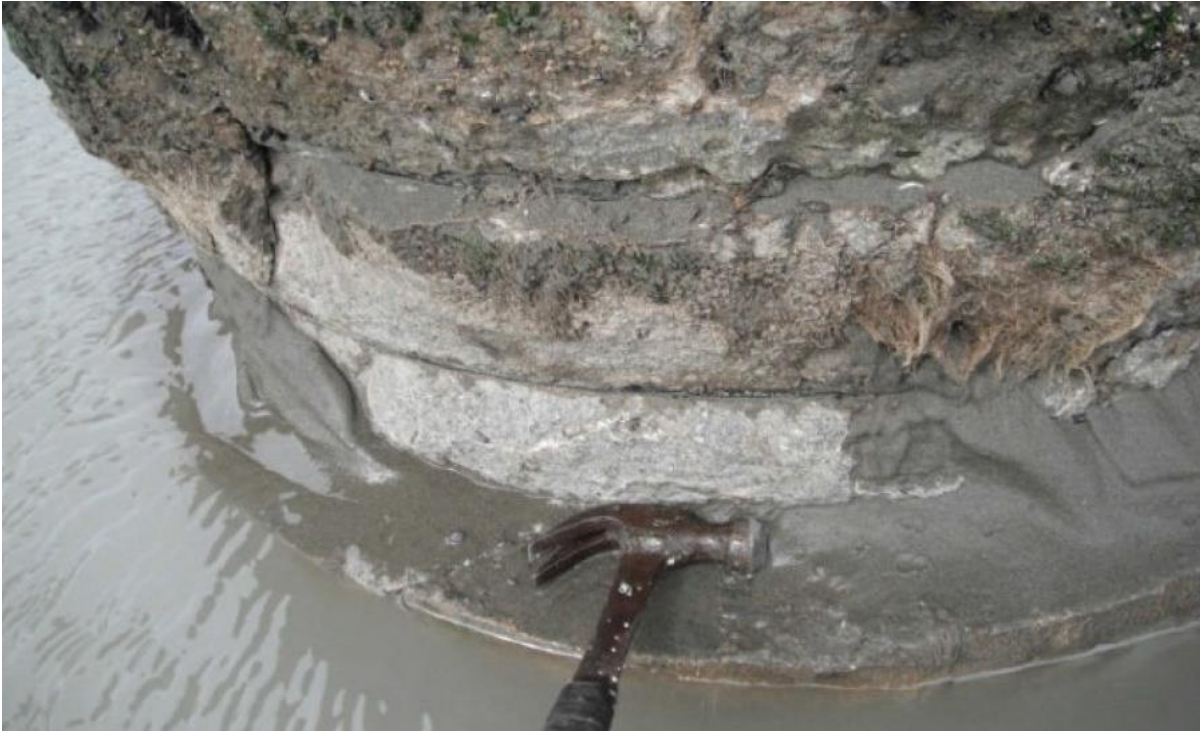
Photo showing the damage to one of the Pier Columns
