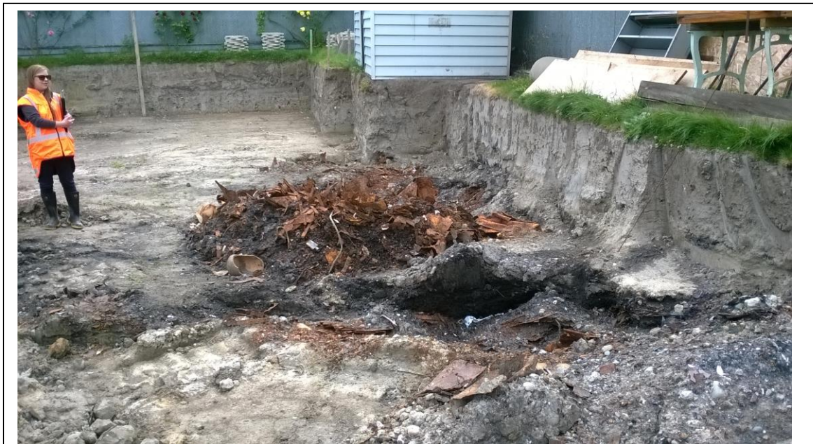
Discovery of a previously unidentified historical rubbish pit, on a residential land repair site, Beckenham.
