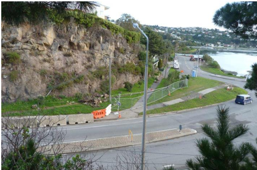
Massey Rebuttal Appendix 1 Figure 2b: 8 Balmoral Lane, 21 June 2011, after the 13 June 2011 earthquake – note boulders at the slope toe. Photograph taken by M. Yetton, Geotech Consulting Ltd.
