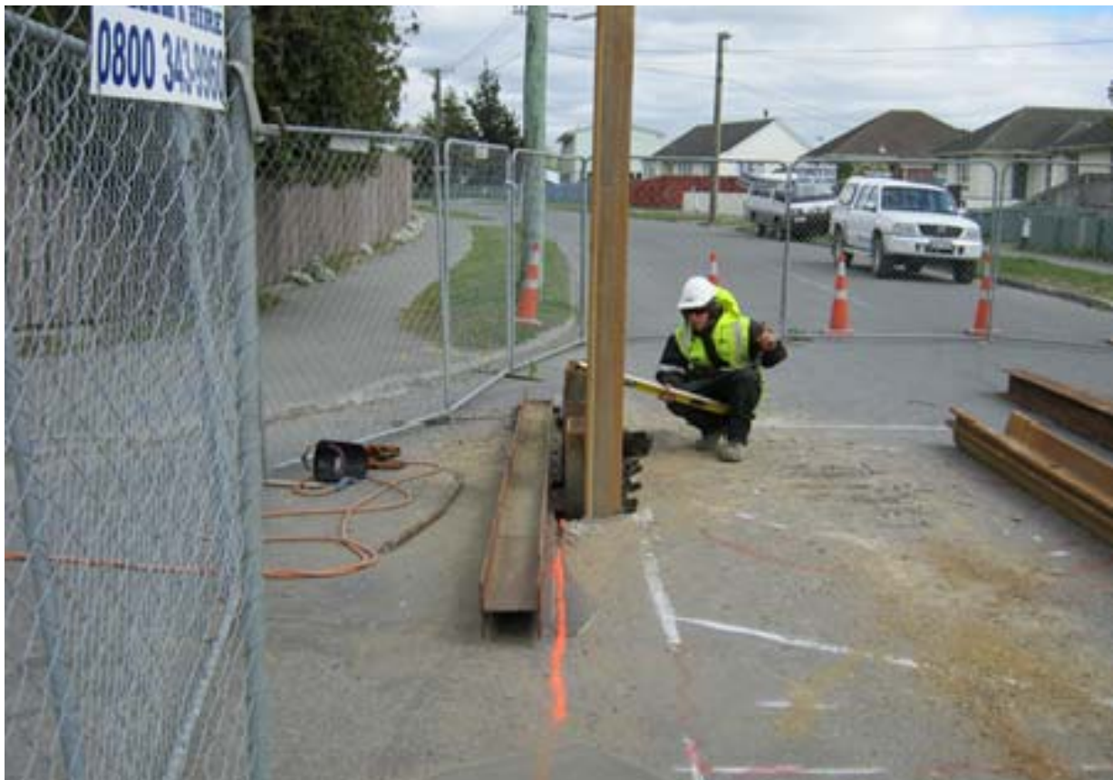
Sheet piling in Eureka Street for connection to the sewer replacement in Rowan Avenue, Aranui
