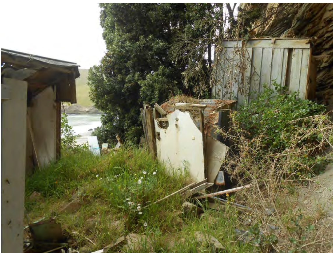
Destruction caused by rockfall debris hitting rear of bach at No.63 Hobsons Bay
