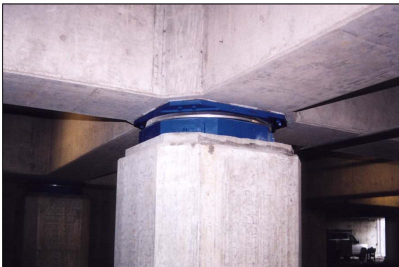
Figure 13 A friction bearing within the lower levels of a car-parking garage – note robust ground floor roll over beams.
