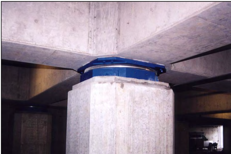
Figure 13 A friction bearing within the lower levels of a car-parking garage – note robust ground floor roll over beams.
