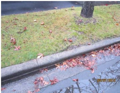
Photo 4 - Crack to kerb and channel
